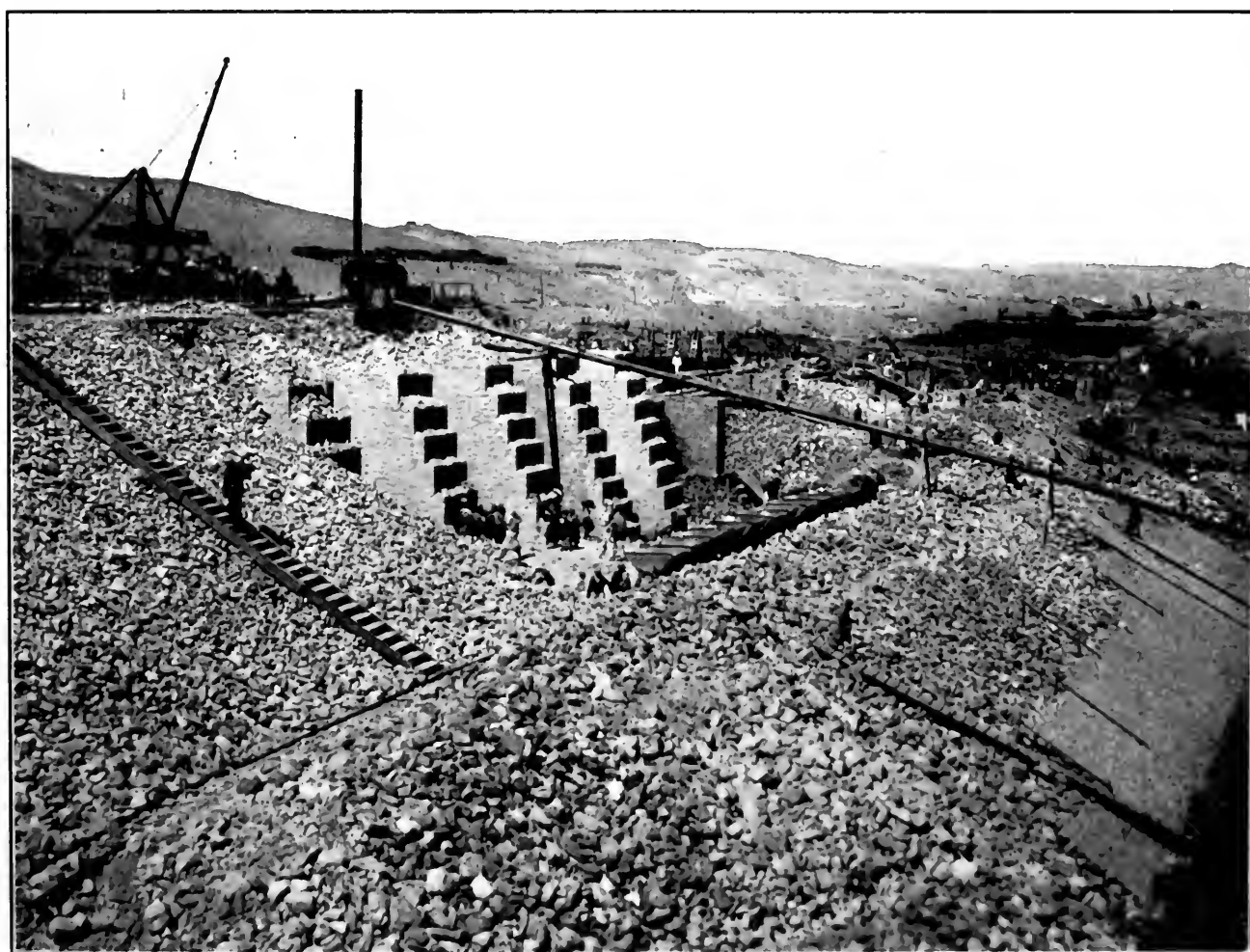
INCREASING THE HEIGHT OF THE ASSUAN DAM BY 16 FEET TO ENLARGE THE ALREADY IMMENSE RESERVOIR SO THAT IT WILL HENCEFORTH CONTAIN 2 BILLION TONS OF WATER, MAKING A LAKE 151 MILES LONG
